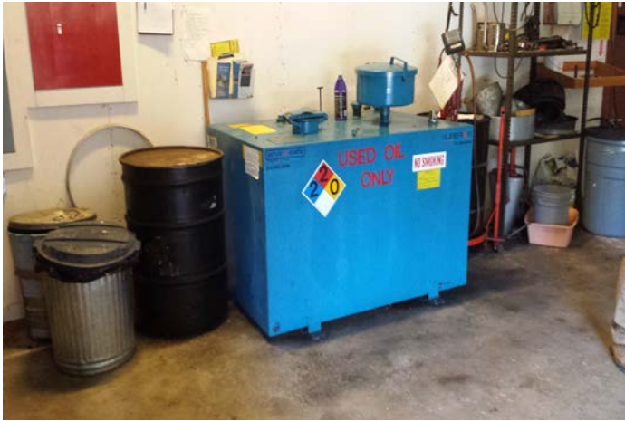
Photo 7: View of waste oil containment inside Apparatus Building.
