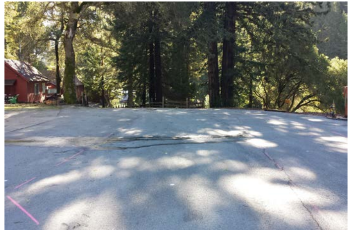
Photo 4: View of paved parking area adjacent to Apparatus Building. Leach Field is located below pavement.
