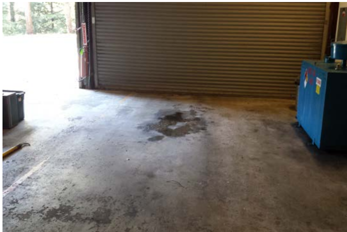
Photo 13: View of minor hydrocarbon staining inside Apparatus Building
