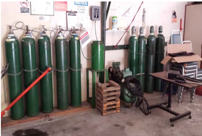
Photo 11: View of onsite oxygen tank storage inside Apparatus Building.
