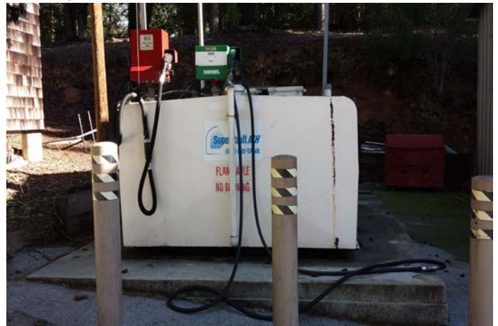
Photo 6: View of Aboveground Storage Tank adjacent to Apparatus Building.
